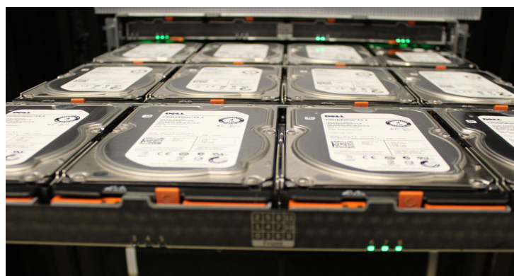
Figure 2. The CI-WATER storage array housed in the research computing area within the University's Downtown Data Center. Photo by Sam Liston
